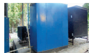
Water Chilling Facility
