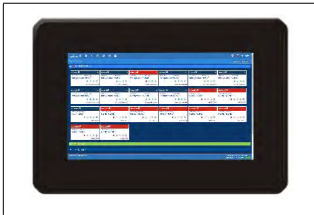
Figure 7-18 - Supervisory Controller Display
